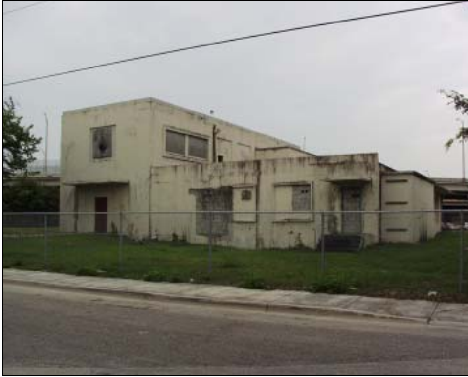
Figure 1: Front and South Elevations, Facing Northeast Photograph taken by Amy Streeleman, August 2002
